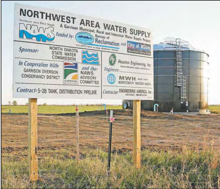
A reservoir tank west of Minot, shown May 28, was completed this spring for the Northwest Area Water Supply project as part of installing a waterline from Minot to Berthold.
