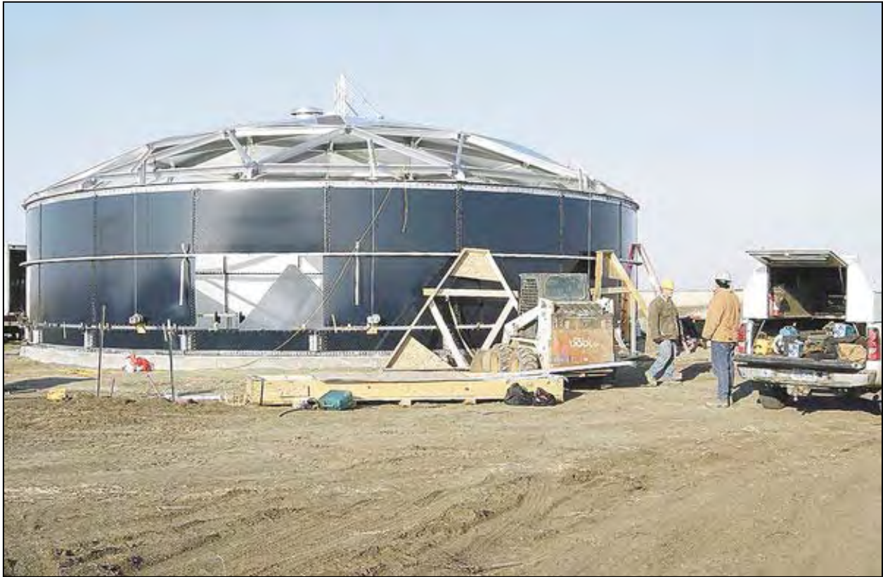
Contractors work Tuesday on erecting a reservoir tank at the top of Speedway Hill, west of Minot, that will be part of the pipeline system delivering NAWS water to Berthold.
