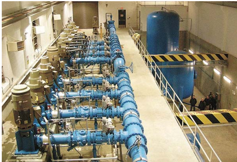
The pipes and pumps at left will serve Minot and the NAWS system. The tanks at right are tanks used to protect against pressure surges. Equipment vendors and engineers were going over the operation with state and city workers Wednesday.
